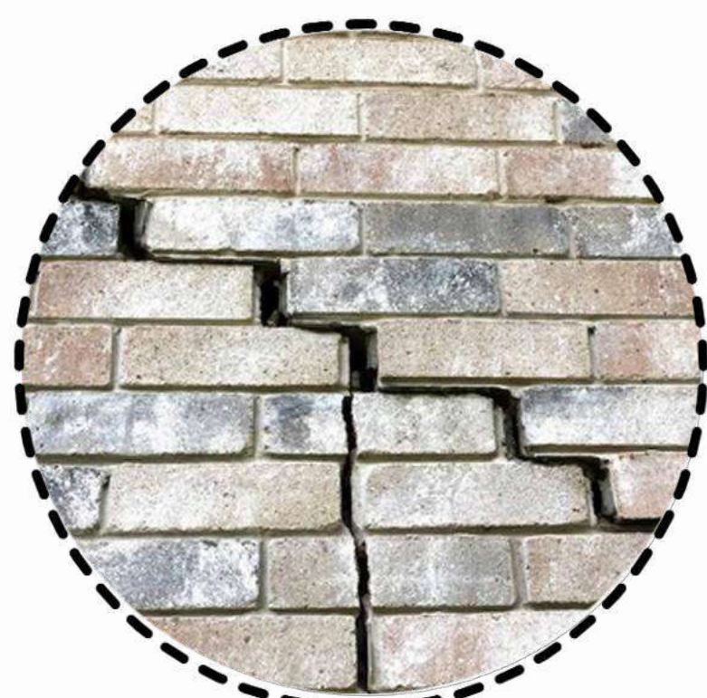
BRICK STAIRSTEP CRACK
