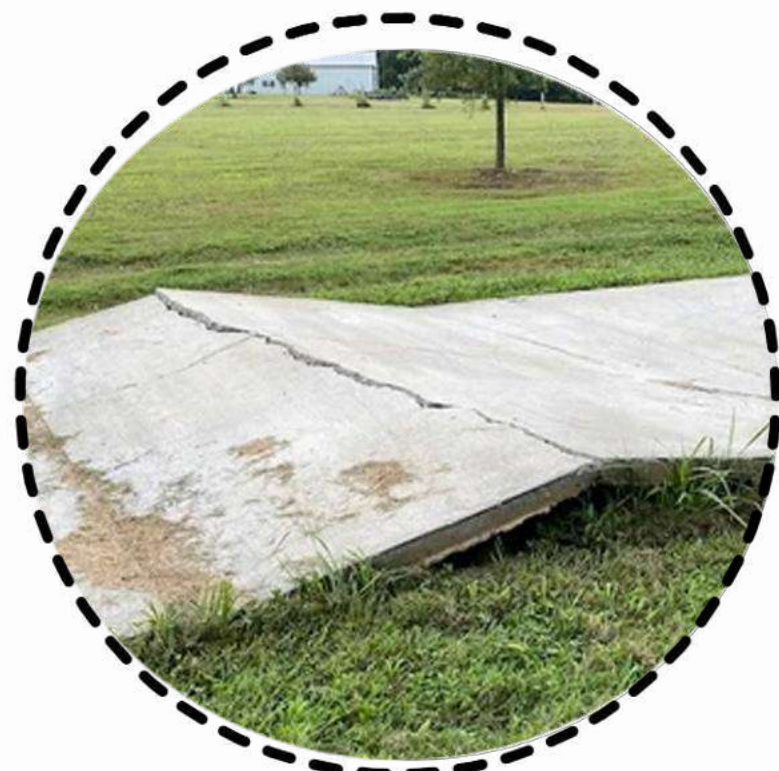
HEAVING CONCRETE CRACK
