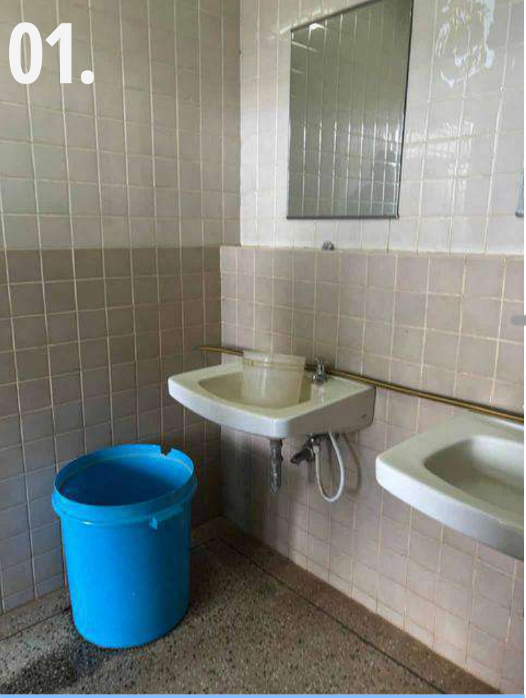
VISIBLE DEFECTS INCLUDE MISSING FAUCETS AND EXPOSED PLUMBING. WALL TILES SHOW SIGNIFICANT STAINING AND DISCOLORATION. A LARGE BLUE BUCKET SUGGESTS POSSIBLE DRAINAGE ISSUES OR WATER SUPPLY INCONSISTENCIES.
