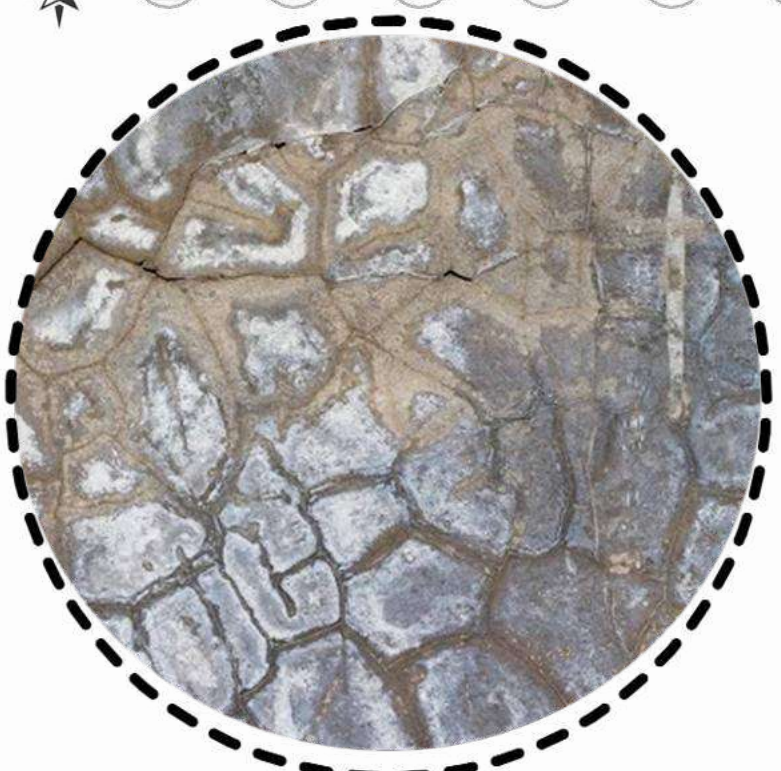
CRUSTING CRACKS CONCRETE
