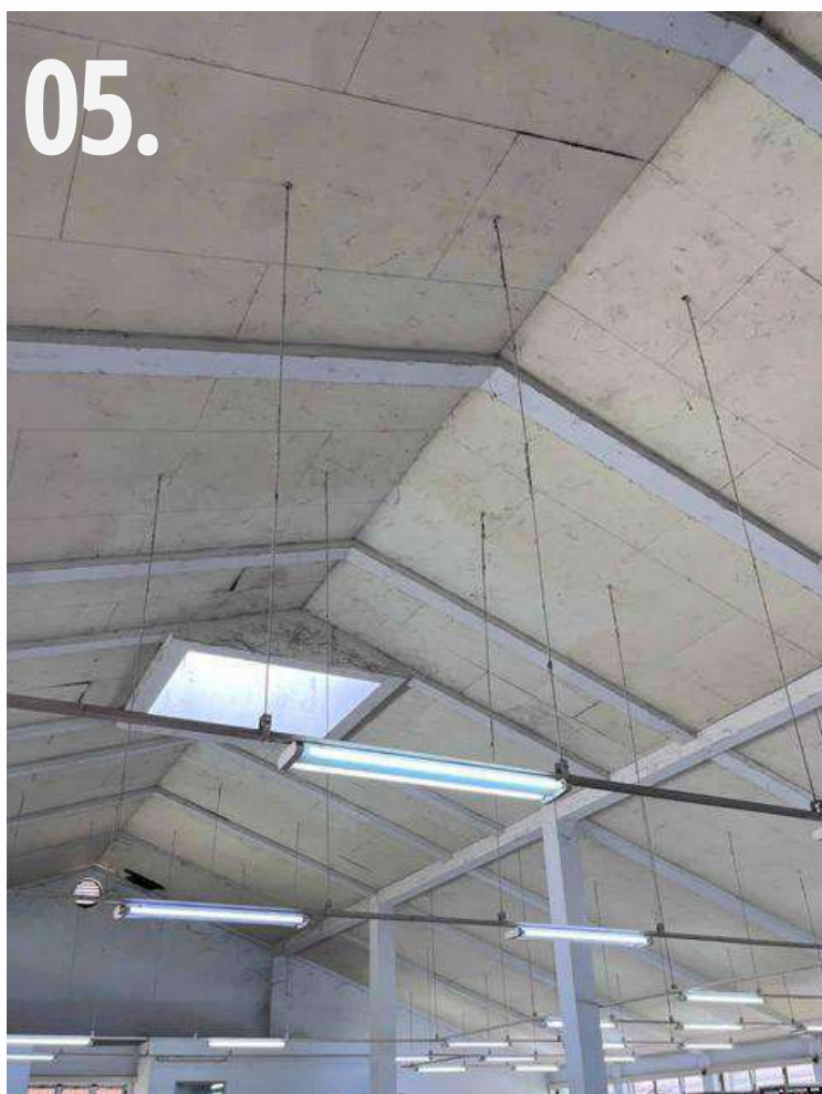
SEVERE WATER SEEPAGE THROUGH DARK STAINING AND MOISTURE PATTERNS ON THE CONCRETE SOFFIT. SUSPENDED FLUORESCENT LIGHTING FIXTURES ARE POSITIONED DIRECTLY BENEATH THESE DAMP AREAS, INDICATING A HIGH-RISK ELECTRICAL HAZARD.
