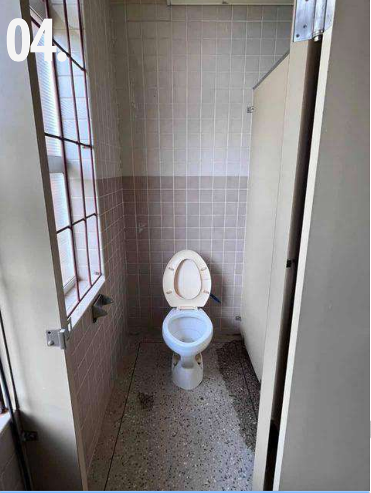
THE TOILET LACKS A CISTERN/FLUSHING MECHANISM. NOTABLE FLOOR DETERIORATION AND DARK STAINING ARE PRESENT ALONG THE PARTITION BASE. THE WINDOW LACKS PROPER GLAZING, AND THE TOILET PAPER HOLDER IS DAMAGED.
