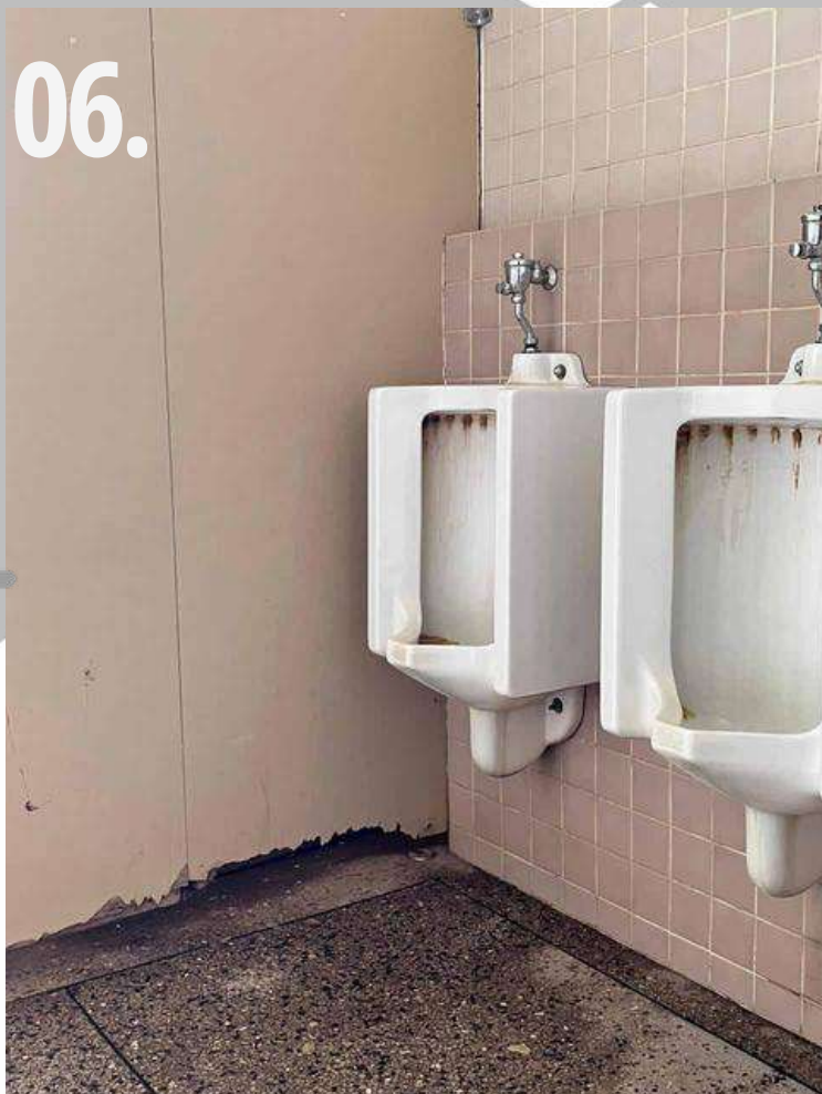
THE URINALS EXHIBIT HEAVY SURFACE STAINING AND BROWN SCALE BUILDUP, PARTICULARLY AROUND THE RIM AND SPREADER. THIS INDICATES PROLONGED LACK OF MAINTENANCE AND POTENTIALLY MALFUNCTIONING FLUSH VALVES.
