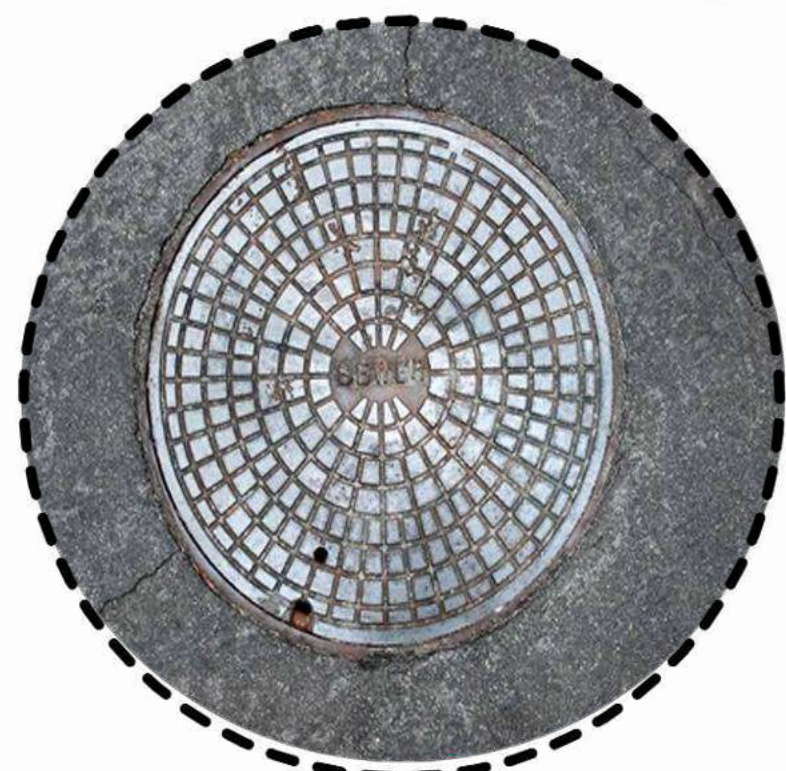
RE-ENTRANT CORNER CRACK
