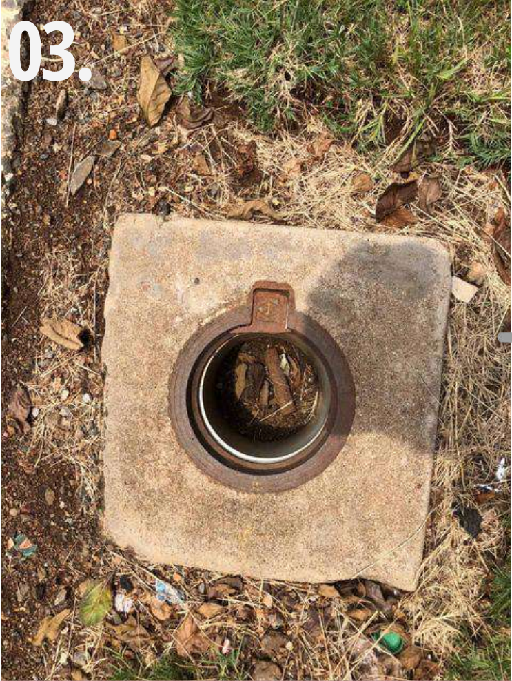
THE DRAINAGE OPENING IS MISSING ITS PROTECTIVE COVER, LEAVING THE PIPE EXPOSED. DEBRIS AND ORGANIC MATTER HAVE ACCUMULATED INSIDE, CAUSING A SIGNIFICANT BLOCKAGE THAT LIKELY IMPEDES WATER FLOW.
