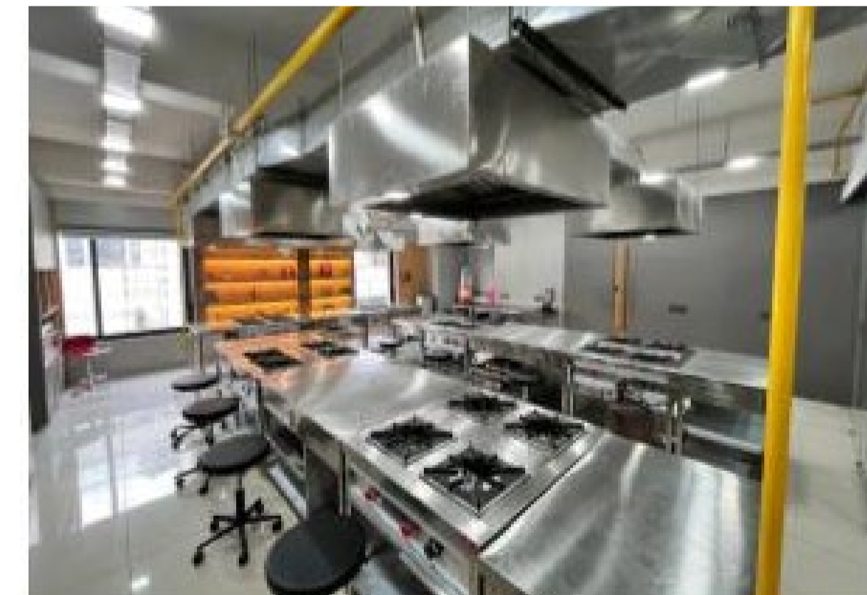
The culinary studio is a fully equipped hot kitchen with individual workstations, chimneys, stoves, washing units, switchboards, and gas pipelines, supporting hands-on training for 15–20 people simultaneously.
