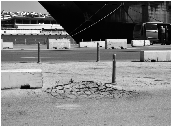
Openings in asphalt
