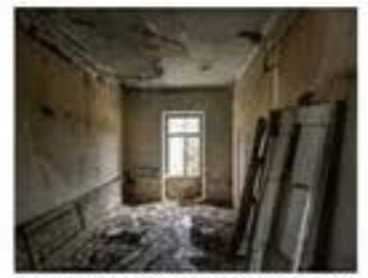
Decay photo (from image_1)
