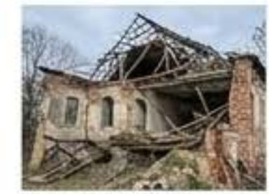
Decay photos (image_1)
