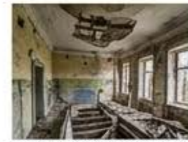
Decay photo (from image_1)
