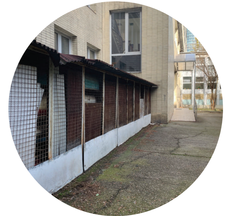
DETERIORATION OF FACADES OF FACULTY BUILDINGS
